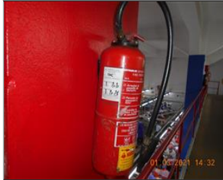
Photo of fire safety equipment fire extinguisher.JPG
