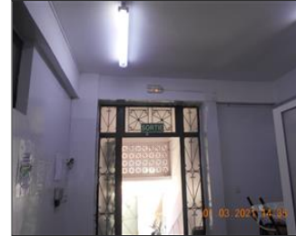
Photo of fire safety equipment emergency exit.JPG
