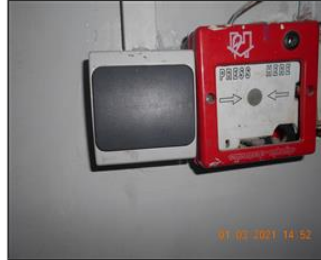
Photo of fire safety equipment Alarm button.JPG
